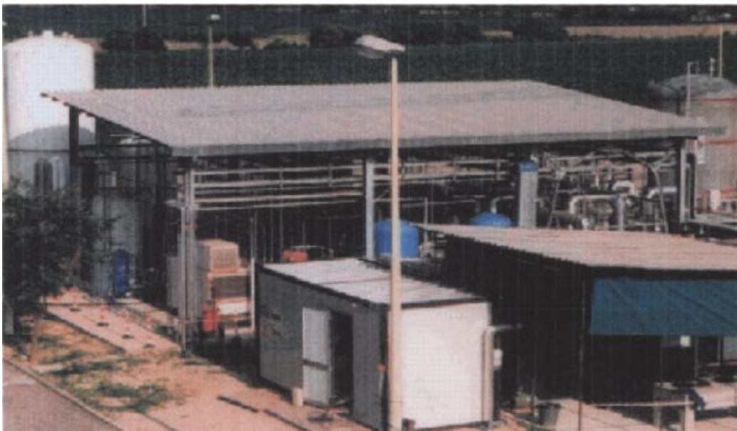
Fig. 2 Proof of concept power plant Ansaldo Fuel Cells MCFC
